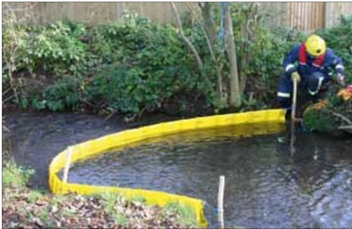
Sequence for river boom deployment. Note the 'tick' shape that moves the spill product towards the bank where flow is slower and it can be more easily recovered.
