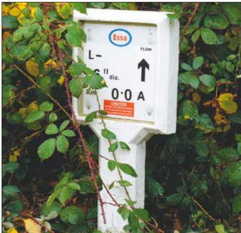
Oil pipeline marker post.
