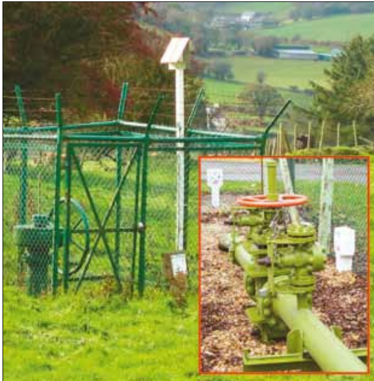
A typical remote valving location. FRS crews may be asked to operate such valves in an emergency so must know their location.
